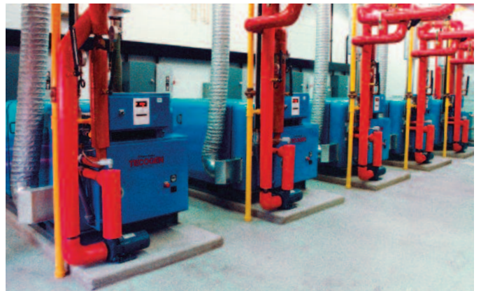
Installed Tecogen cogeneration modules. Photo courtesy of Tecogen, Inc.
